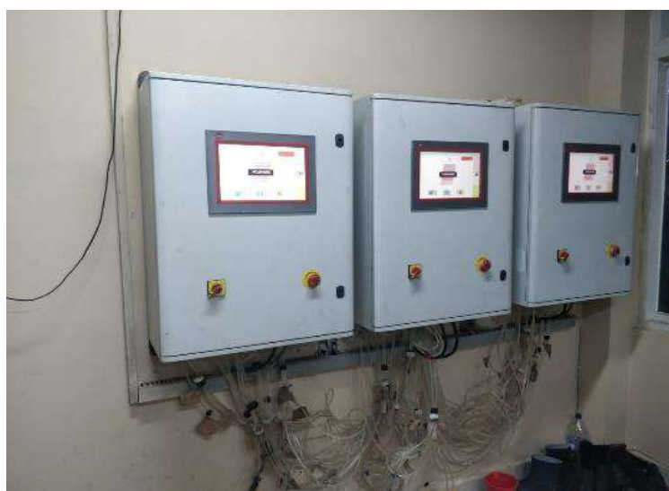
Picture 5: AQUAMIX - Water mixing equipment to control the water and dosing into the system
